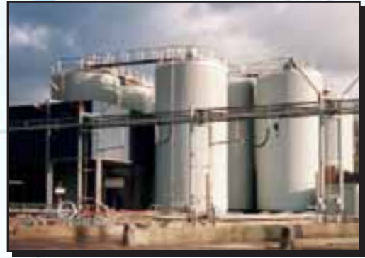
Level measurement on storage tanks
